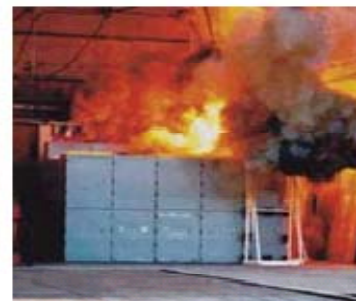
Internal arc failure
