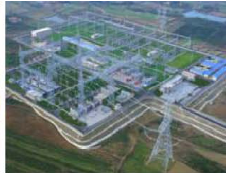
China 1100kV projects
