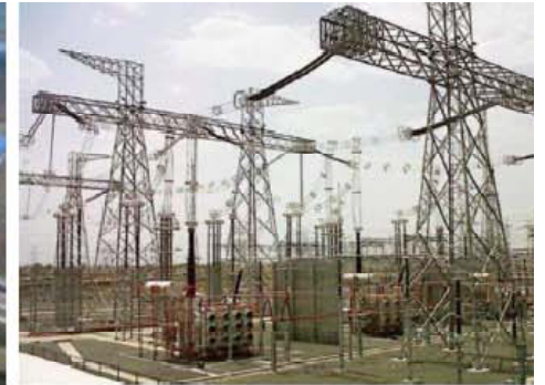
India 1200kV testing field
