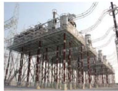
1100kV Series-capacitor bank
