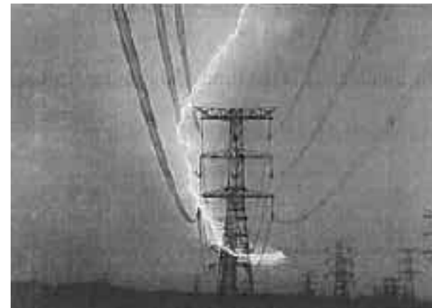
Lightning stroke to Transmission lines
