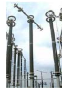
800kV DC Bypass Disconnectors
